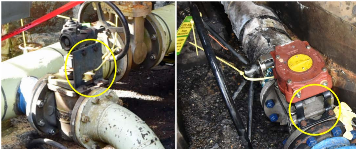
Figure 8. Two of several designs of gearbox support brackets (yellow circles) used at the Baton Rouge refinery. These specific brackets attach to the valve body flange – they are not among the approximately three percent of valves in the alkylation unit that attach the gearbox support bracket using the same four vertical bolts that secure the pressure-retaining top-cap.
